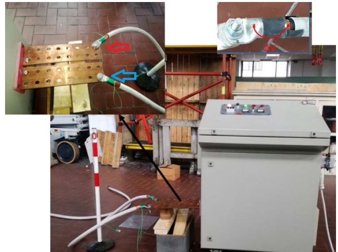
Fig.3. Measurement setup with zoom of the connection between the cable lugs and the bars and of the place where voltage measurements have been made.
