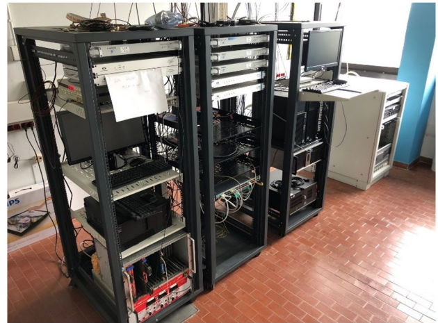
Fig. 3 E3F installed, calibrated and operated at INRIM Radio Navigation Laboratory. E3F is the first left-side rack. From top to bottom, the distribution section, the acquisition section (with the SR620 TIC and, not visible, the Raspberry Pi 3 B+ and GR03) and an EEE telescope crate containing the Spectracom TSync and Trimble SMT 360 single-frequency receivers. GTRB belongs to the Time Laboratory measurement system, while INR5 is installed in the picture central rack
