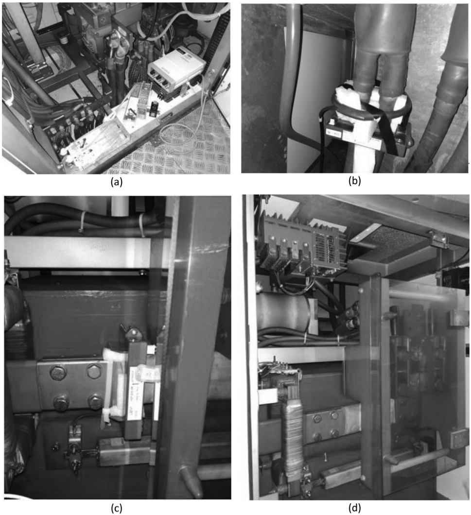
Fig. 6. Installation of the DAS and transducers: a) voltage transducer and supply systems for the active sensors and the DAS; b) Rogowski coil for the i_r measurement; c) HOP sensor for the i_p measurement; d) DAS.
