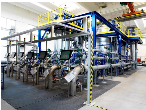
Figure 3: The flow Calibration plant at Hemina Laboratory
