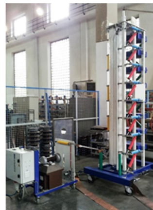
Fig. 3. HAEFELY SGSA 800/40 impulse generator.
