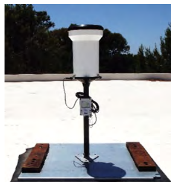
(b) Tipping-bucket gauge installed in field
