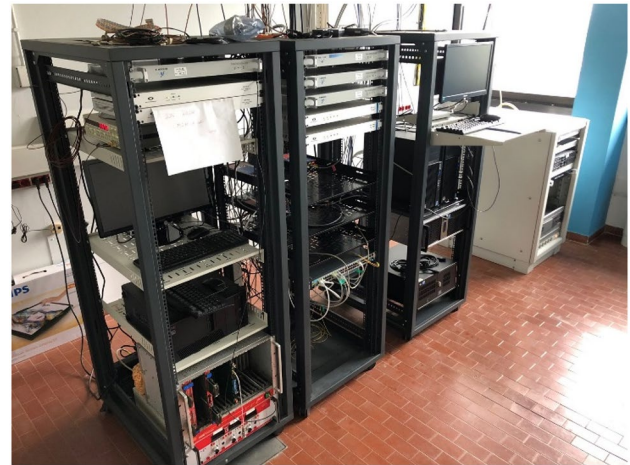
Fig. 3 E3F installed, calibrated and operated at INRIM Radio Navigation Laboratory. E3F is the first left-side rack. From top to bottom, the distribution section, the acquisition section (with the SR620 TIC and, not visible, the Raspberry Pi 3 B+ and GR03) and an EEE telescope crate containing the Spectracom TSync and Trimble SMT 360 single-frequency receivers. GTRB belongs to the Time Laboratory measurement system, while INR5 is installed in the picture central rack
